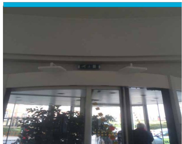
Figure 4: RFID readers installed at doors in the hospital.
